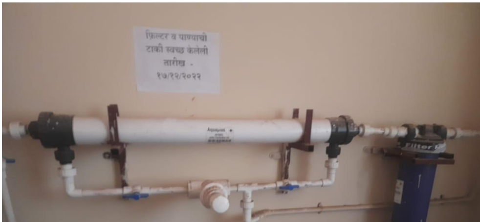
Advanced water filter unit
