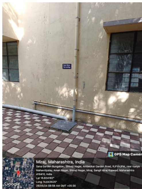
Rainwater collection pipe for Ground water recharging:
